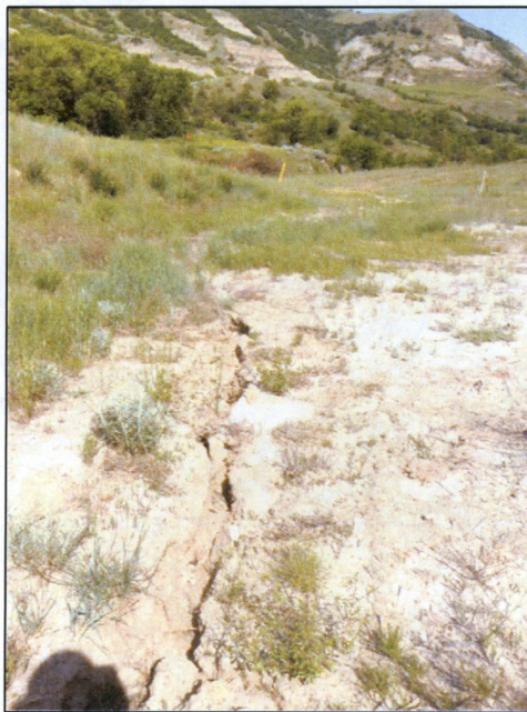
Photograph 8. Incising stream channel across eastern edge of ROW fill. View to northwest.
